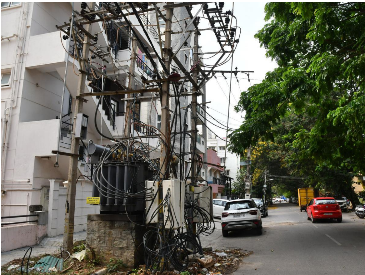
An unguarded transformer in Bengaluru. | Photo Credit: FILE PHOTO
