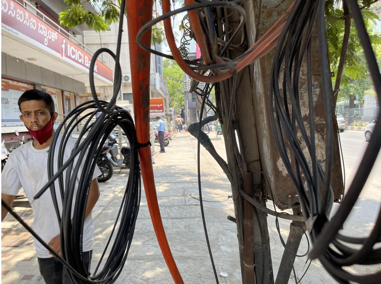
A wire dangerously hanging on a footpath in Bengaluru. | Photo Credit: K. MURALI KUMAR
